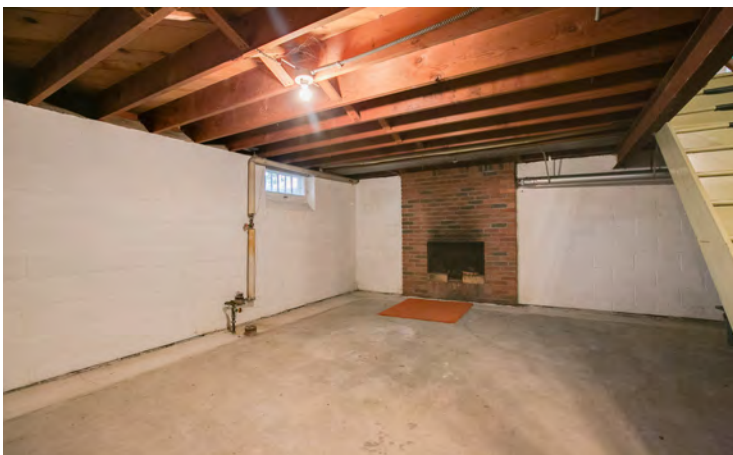
The basement is fully drain tiled, with a second fireplace and quarter bath... dry and ready for finishing.
